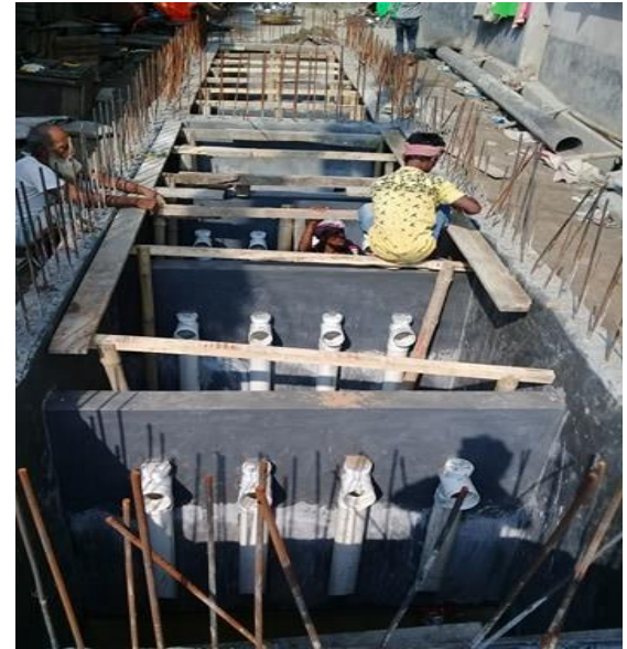
Baffled wall & piping
