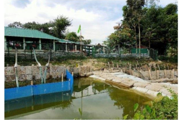
Roikong Canal Intake Pipe
